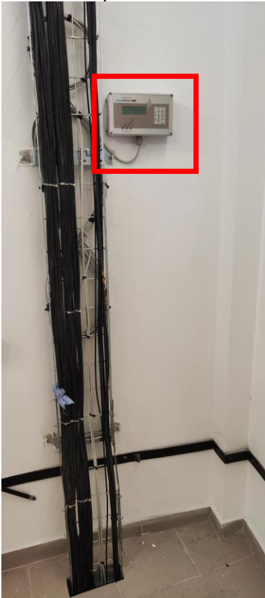
Central operator panel TABD
